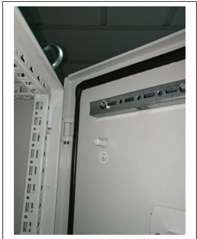
Fig. 11: Connections for the earthing cable
