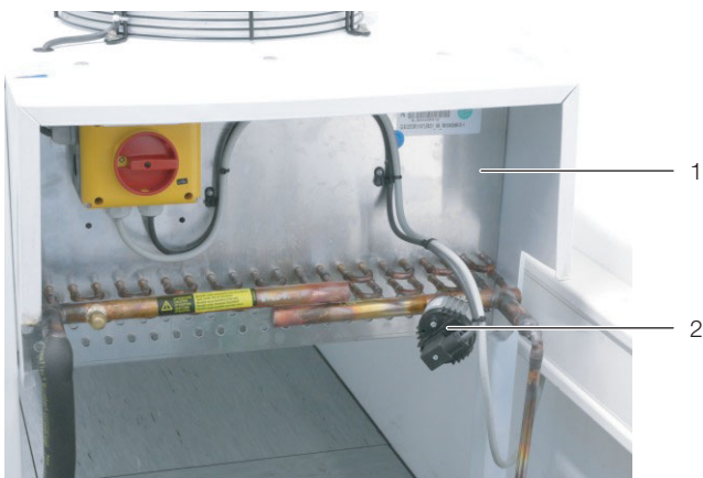
Fig. 27: Pressure switch on the condenser
