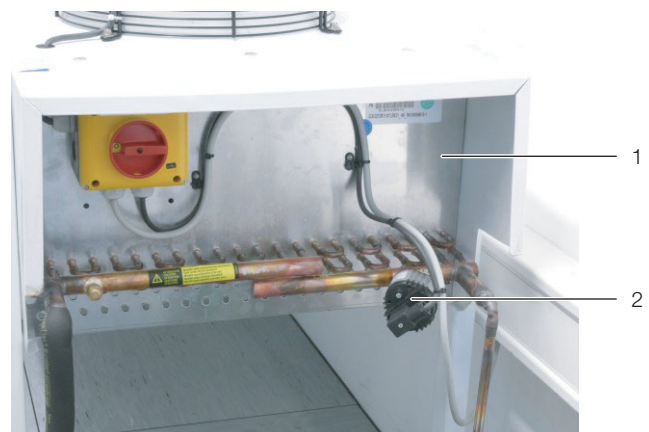
Fig. 27: Pressure switch on the condenser
