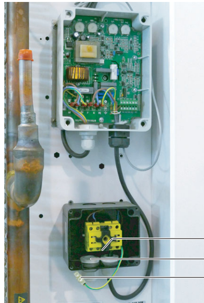
Fig. 27: Electrical connection on the external condenser
