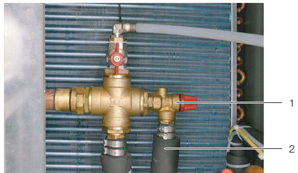
Fig. 24: Safety valve at rear
